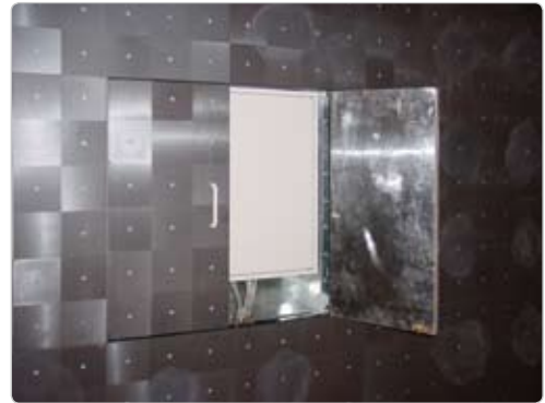
Electrical distribution box access from inside
