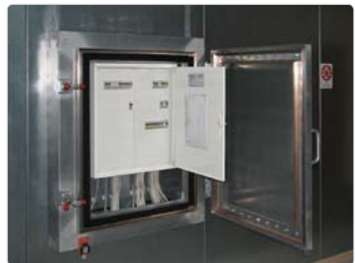
Electrical distribution box access from outside
