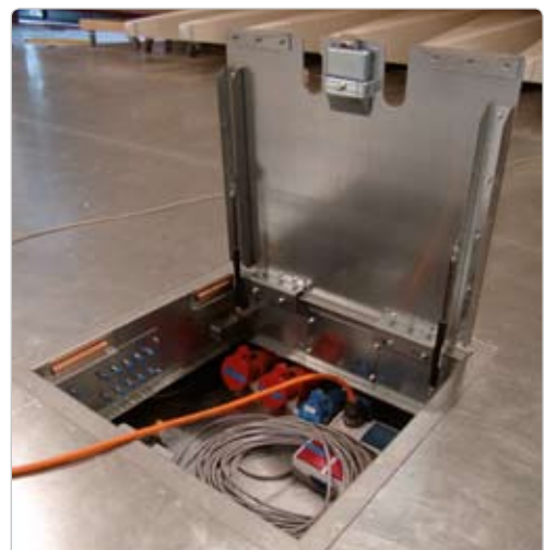
Outlet box in raised floor
