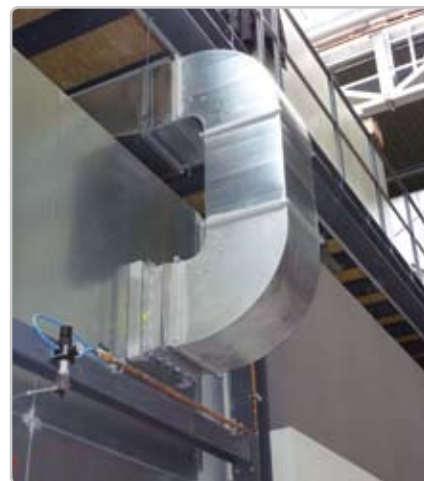
Direct connection to air conditioning system
